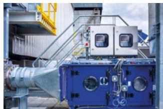
Dynamic pressure/ psychrometry/ temperature/airflow/ACR** regulation in air handling units and ductworks
